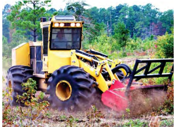
Gyro Trac at work on 40 acres of the Colleton County Commerce Center Park
